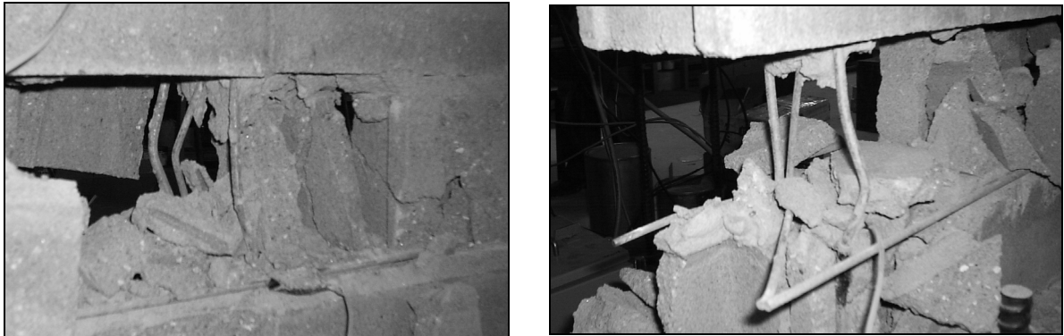
Figure 12: Buckling of the reinforcement because of the high compression stresses.
