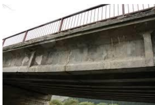
Figure 2 Crack in the middle of span due to corrosion of prestressing steel before the collapse in village Podbiel, Slovakia.
