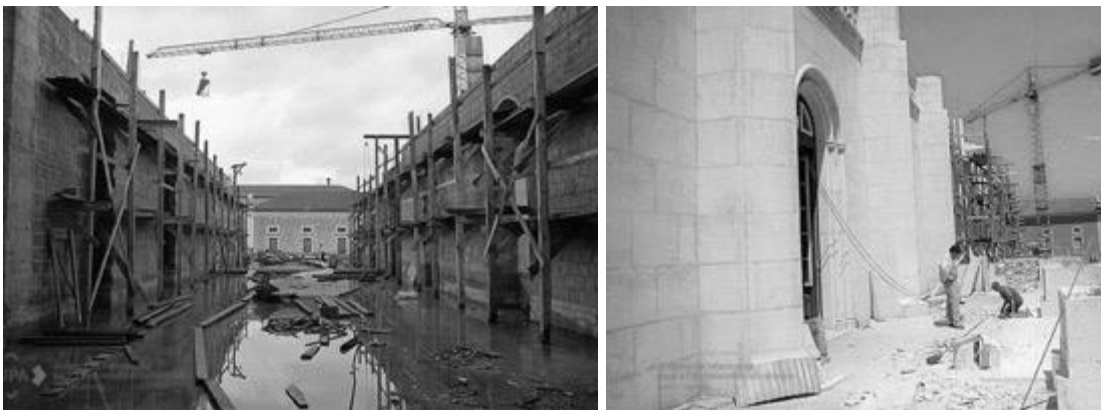
Figure 11: left: photograph of the first floor of the North wing mid-construction, c. 1984, Foto 504317, © IHRU/SIPA; right: photograph of the façade of the North wing mid-construction, c. 1984, Foto 00504325, © IHRU/SIPA.
