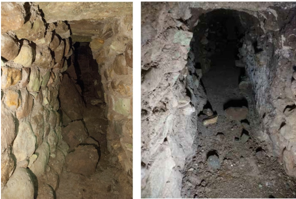
Fig. 5. Examples of local collapses at the interface between lined and unlined tunnels – left – and in an unlined tunnel – right [12].
