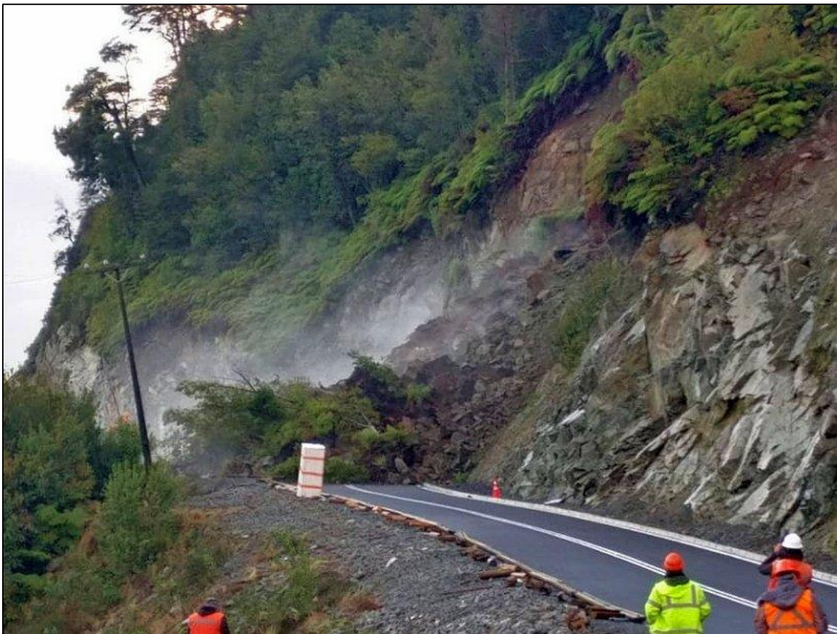
Figure 34 To modernize and pave Route 7, several cuts were made on the slopes of the hill, removing rocks and sediments. This action exposed several outcrops but also generated significant instability on the slopes. The stabilisation of the road may result in the permanent modification of the landscape. For instance, using shotcrete may permanently lose the visibility of some outcrops. Photo: Ruta 7, Chaitén, taken from Diario el Huemul (2018).
