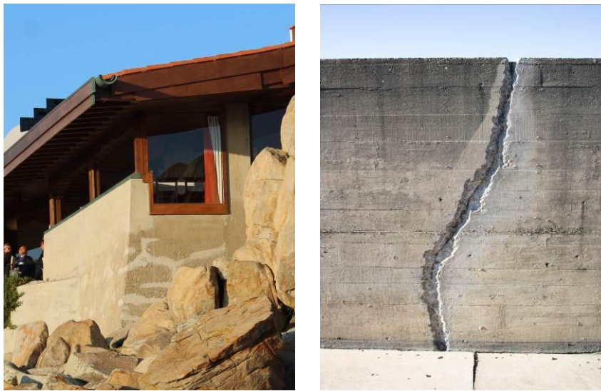
Fig. 4. Concrete repair solution in the Tea House (2019) and Swimming Pool (2019, proposal) (photos by Frederico Barbosa)
