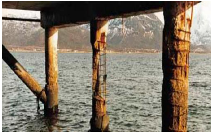
Figure 4 – Photo example of corrosion-induced damage on a reinforced concrete marine structure (Alexander and Nganga, 2014)
