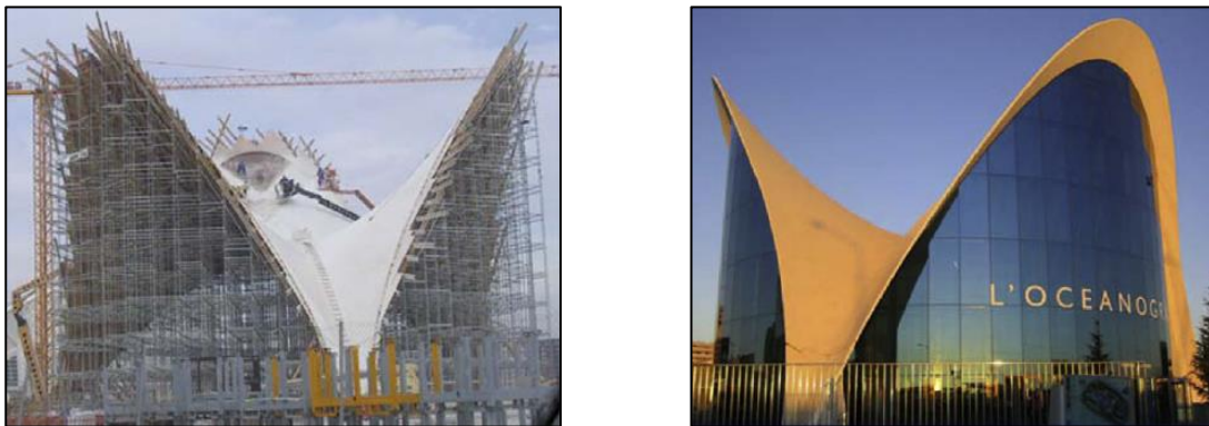
Figure 6 – Under construction and completed shell structure at the entrance of the Universal Oceanographic Park in Valencia, Spain (Tomás and Martí, 2010)
