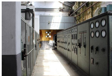
e) Central electric unit
