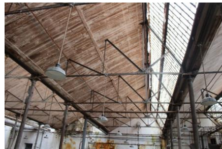
(e) Corrugated steel roof covered by wood paneling in the main rooms
