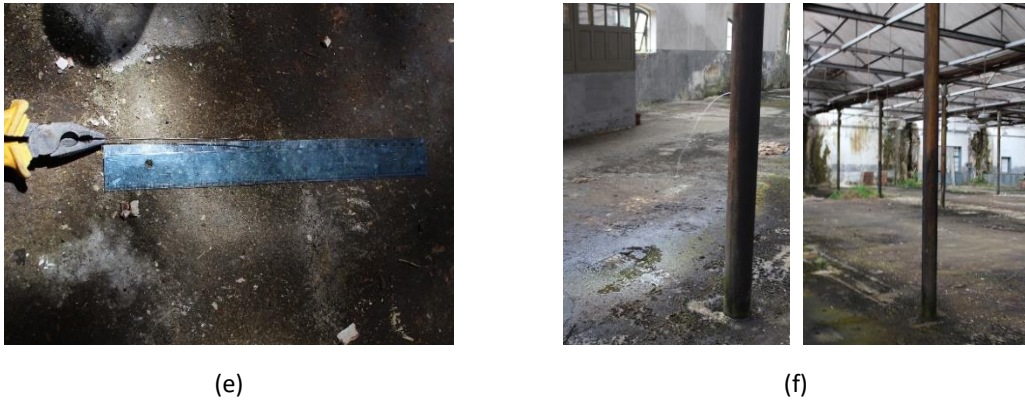
Figure 7 – (a) Location of tested columns; (b, c, d and e) Wall thickness measurement (Bussell, 1997): in-field demonstration of the procedure to measure the column thickness; (f) Water pouring out from the hole drilled and full discoloration of Column 6
