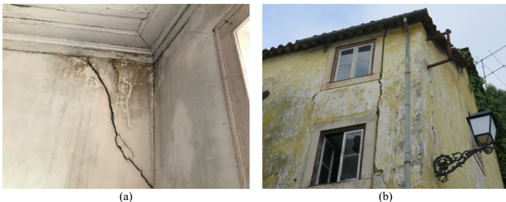
Figure 4. Bad quality connections between orthogonal walls evidenced by diagonal cracks on internal walls (a) and by detachment cracks on the corners (b)
