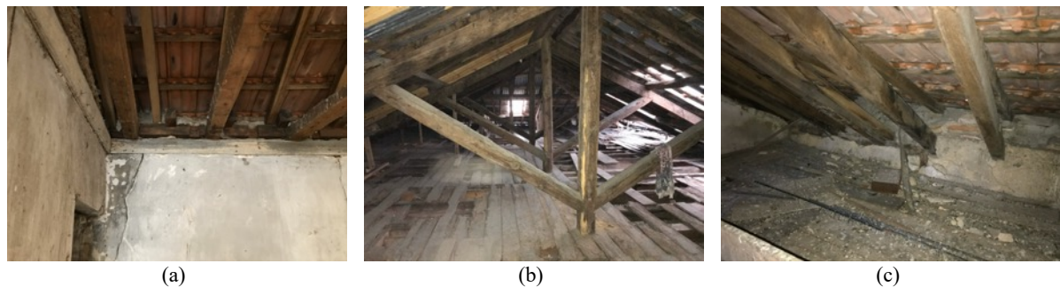
Figure 5. Example of a two-order timber floor with connection to the perimeter wall (a), timber king post truss of a roof (b), mixed masonry-timber perimeter ribbon of the roof (c)
