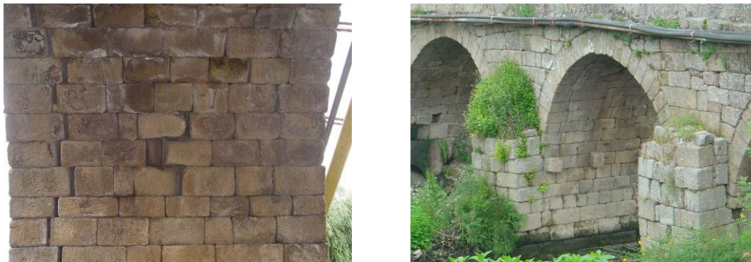
Fig. 7 Examples of damage: longitudinal cracking in the central arch and vegetation and cracks in the downstream cutwaters (downstream view).
