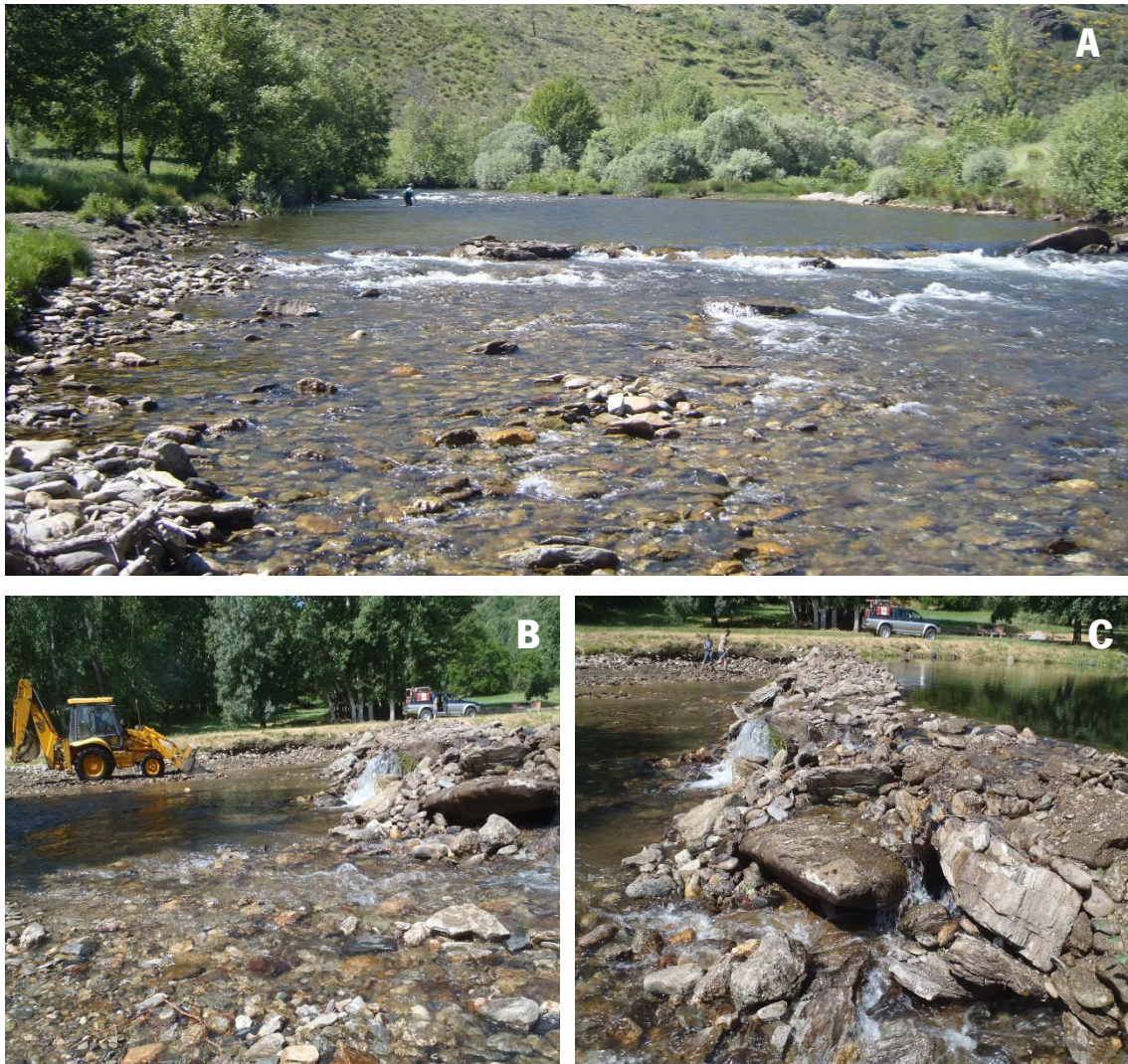
Figure 21 – Before (2012) (A) and after (2017) (B, C) the construction of a weir with the goal of creating an artificial river beach for visitors inside Montesinho Natural Park. Courtesy of Ronaldo Sousa.
