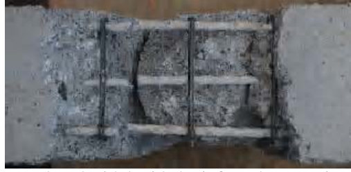
Figure 7 – Beam produced with braided reinforced composite rods after testing
