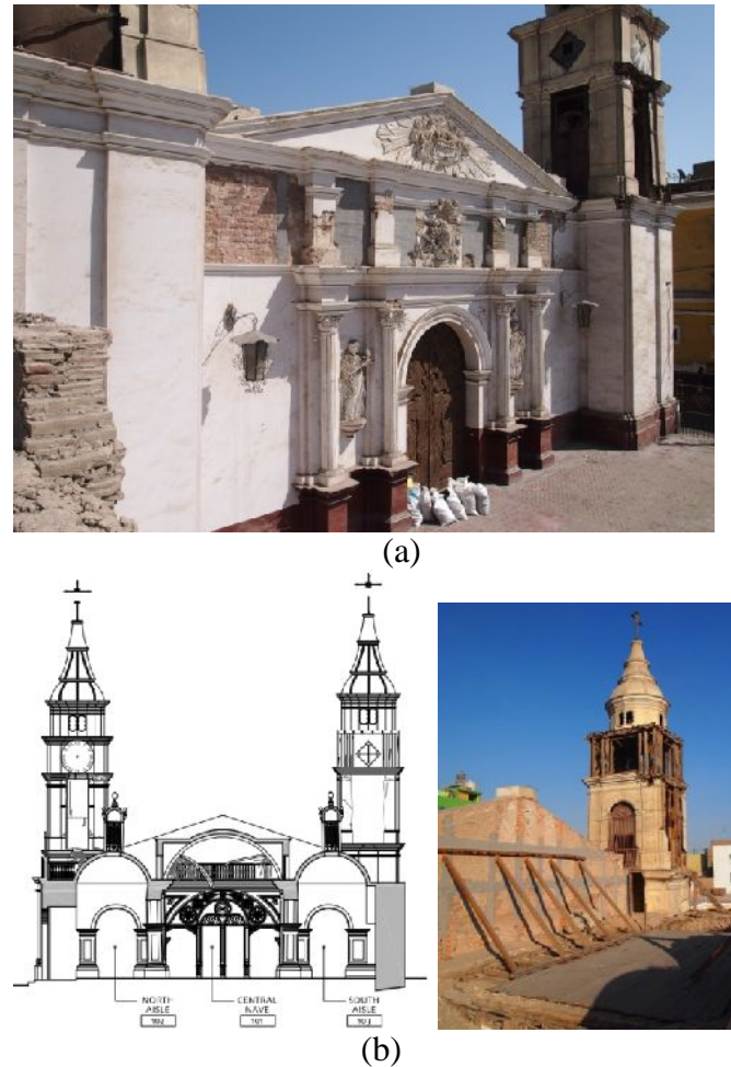
Figure 1. Front façade of the Cathedral of Ica (a); main façade drawing and view of the gable from the back side (b).
