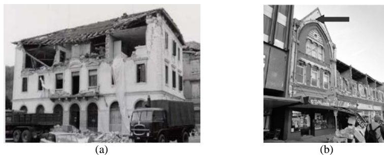
Fig. 7 Examples of out-of-plane collapse mechanism: (a) wall of the top floor [22]; (b) parapet and wall collapse and successful strengthening with ties (arrow) [23].
