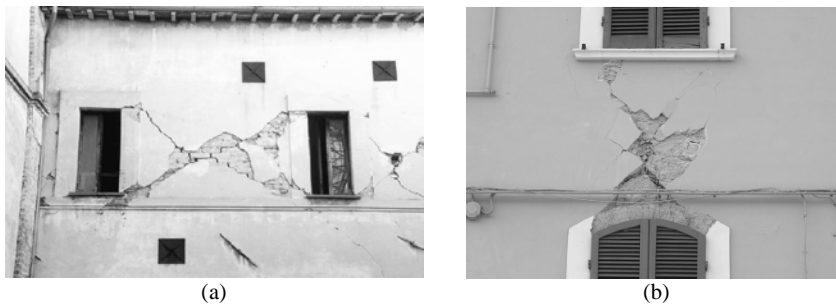
Fig. 6 Examples of shear failure of: (a) piers [20]; (b) spandrels [21].
