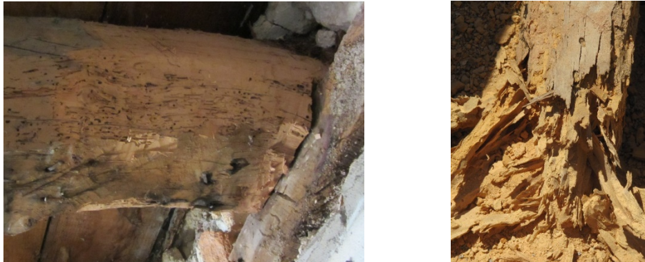
Figure 1. Examples of decayed old timber end beams.
