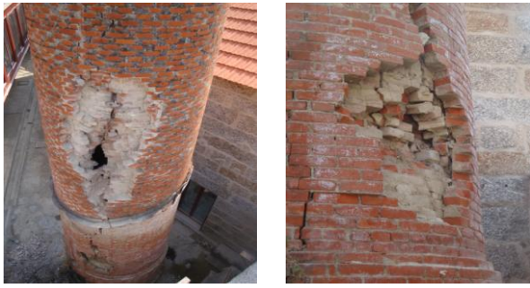
Figure 2. Openings caused by the lightning.
