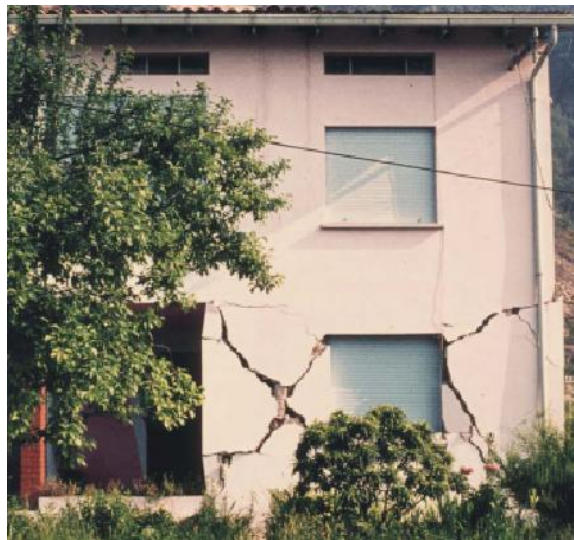
Figure 2.1 - Diagonal crack in masonry walls and loss of corner wall URM masonry' R.C. floors [14]
