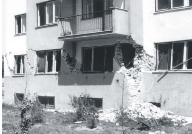
Figure 7.5 - Concentrated damage at the ground floor [39]
