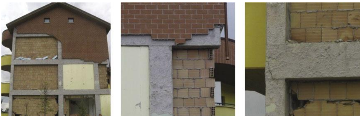
Figure 10. Failing of the exterior leaf due to improper connection [1] L'Aquila.
