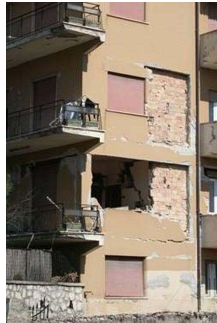
Figure 9. Out-of plane failure, overturning of the external leave or the whole infill [28]. L'Aquila.
