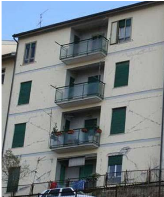
Figure 8. Typical diagonal in-plane cracking of infills [28] L'Aquila.
