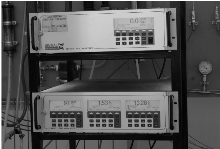
Figure 4 –View of the SIGNAL 9000MGA flue gas analyzer
