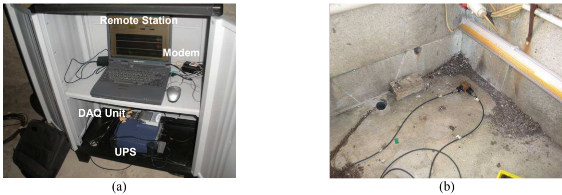
Figure 6: Continuous Dynamic monitoring system setup. (a) Data acquisition station; and (b) measurement node
