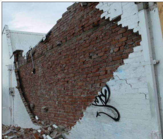
Figure 6: Out-of-plane failure of a single leaf veneer.
