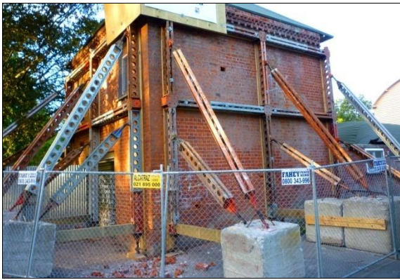
Figure 34: Extensive steel temporary shoring of a URM building following the 4 th Sept earthquake.
