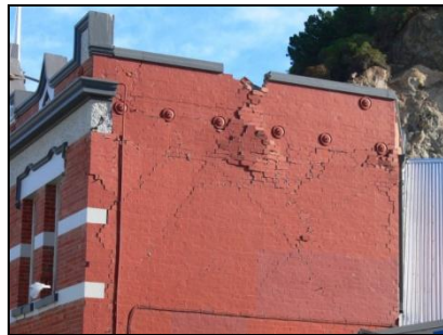
(b) Post-February 2011 – section of masonry on verge of collapse
