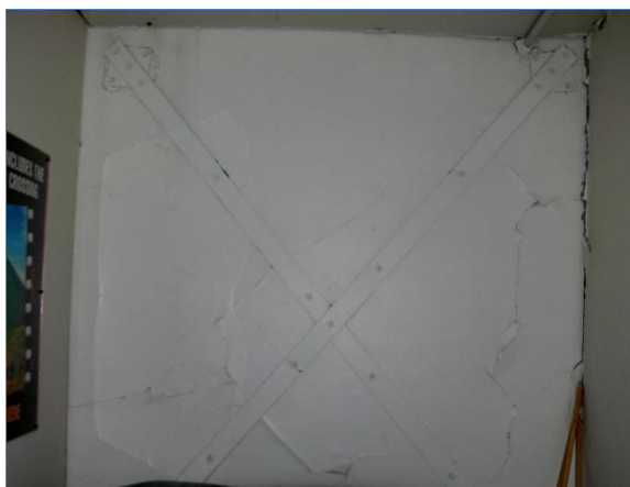
Figure 22: 'X' steel bracing retrofit with extensively cracked masonry.
