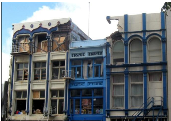
Figure 16: Pounding between three buildings, causing in-plane failure in URM buildings.
