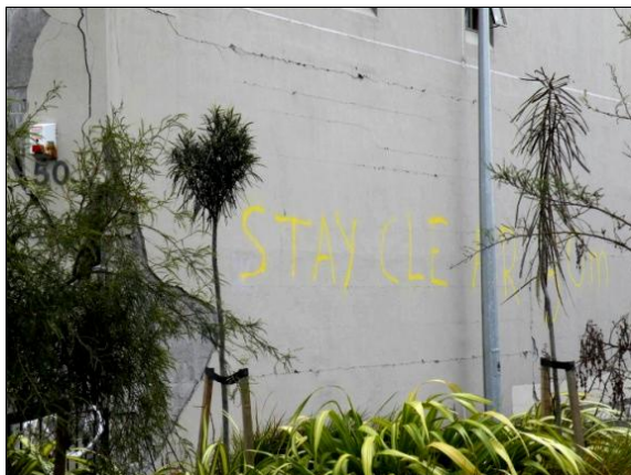
Figure 47: Bed joint cracks indicating yielding of reinforcement across the height of the first floor.
