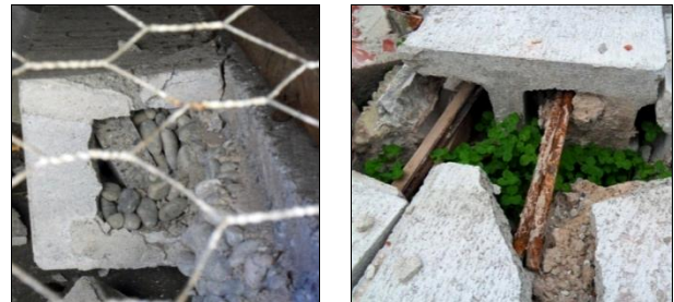
(a) Poor cell grouting (b) UngROUTED masonry cells
