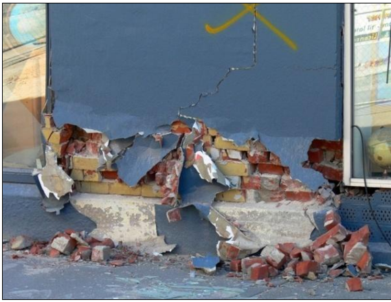
Figure 12: Close-up of toe crushing failure mechanism.
