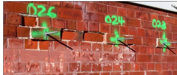
Figure 32: Typical masonry pullout type failure observed.
