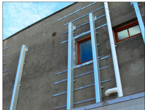
Figure 20: Externally positioned steel strong backs prevented out-of-plane failure of a tall and slender URM wall.
