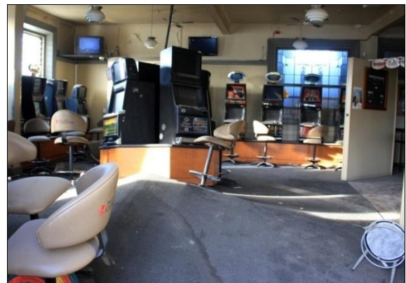
Figure 17: Extreme floor movement due to severe differential ground deformation.
