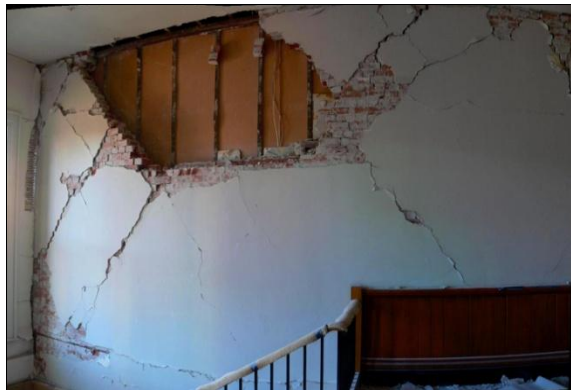
Figure 5: Two-way bending out-of-plane wall failure.
