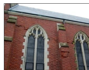
(b) Nazareth's House Church, shear mechanism on the longitudinal walls
