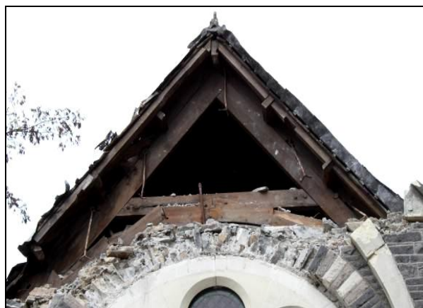
Figure 38: Former Trinity Church, showing details of gable end out-of-plane wall failure.
