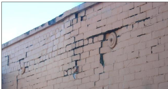
Figure 28: Wide spacing of anchors resulting in horizontal bending failure of masonry.
