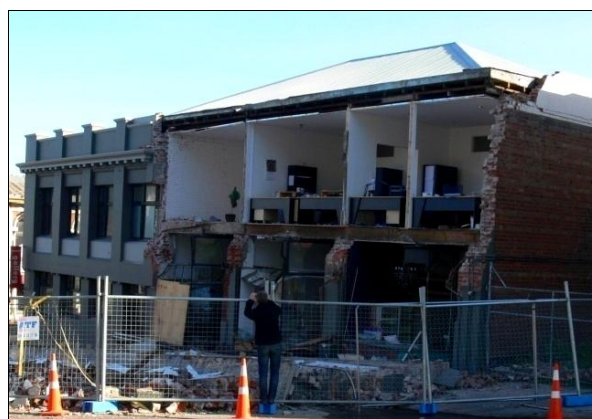
Figure 3: Out-of-plane collapse of parapet and façade, Lyttelton.
