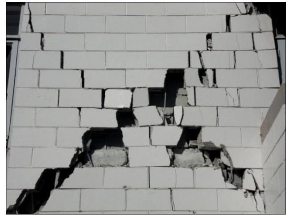
Figure 44: Severe diagonal cracking of RCM cavity shear wall.
