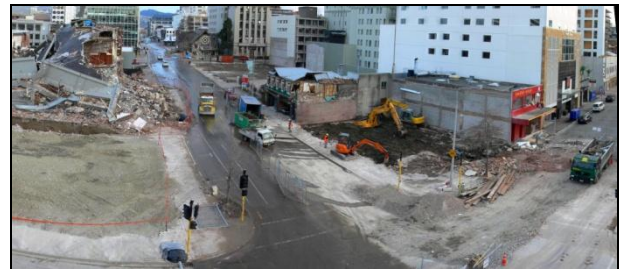
Figure 2: Extensive building demolition following the 13 th June 2011 aftershock.
