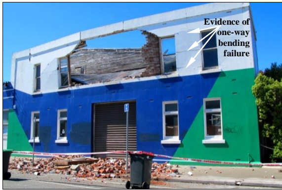
Figure 4: One-way bending out-of-plane wall failure below a concrete ring beam.
