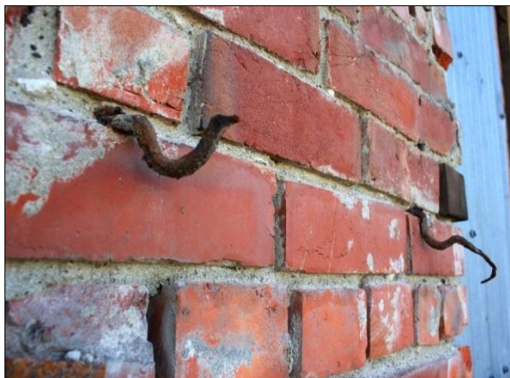
Figure 7: Metal cavity ties in poor rusted condition.
