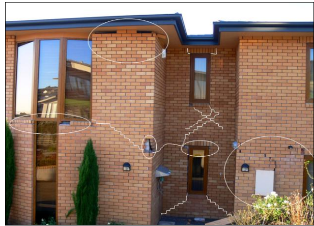
Figure 55: Example of severe veneer damage level.
