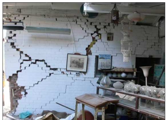
Figure 11: Diagonal shear cracking of unperforated wall.
