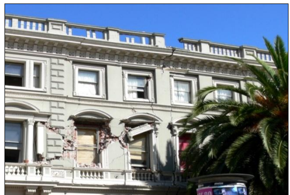
Figure 9: Diagonal shear cracking through piers and spandrels.
