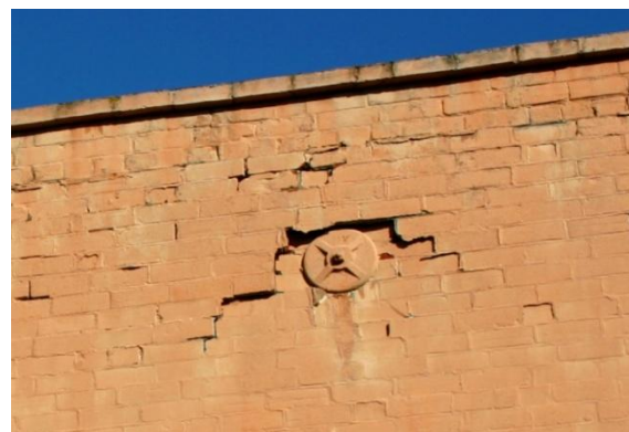
Figure 24: Anchor on the verge of punching shear failure.
