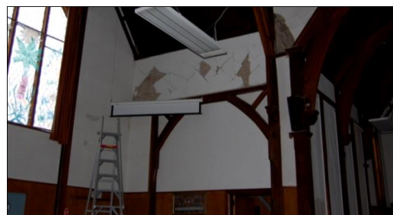
Figure 52: Damage to the internal plaster of St. Paul's Anglican Church, Harewood Road.
