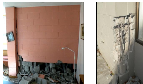
(a) Flexural failure of RCM wall due to spalling and crushing of grout (b) Buckling of unsupported lap-spliced vertical reinforcement
