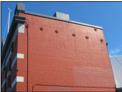
(a) Post-September 2010 – minor visible damage
