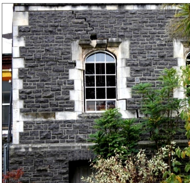
Figure 37: Canterbury Provincial Chambers - diagonal crack through entire south façade of the east annex.
