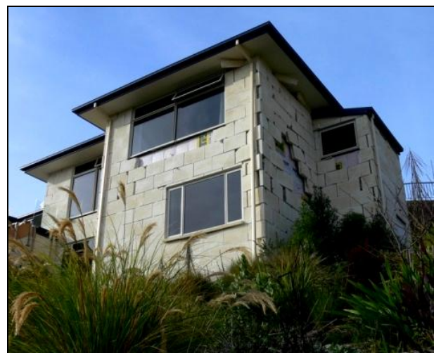
Figure 56: Poor performance of Oamaru stone veneer.
