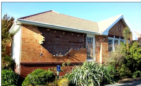
Figure 23: Post June 2011 condition of a veneer layer tied using inserted high strength twisted stainless steel rods.
