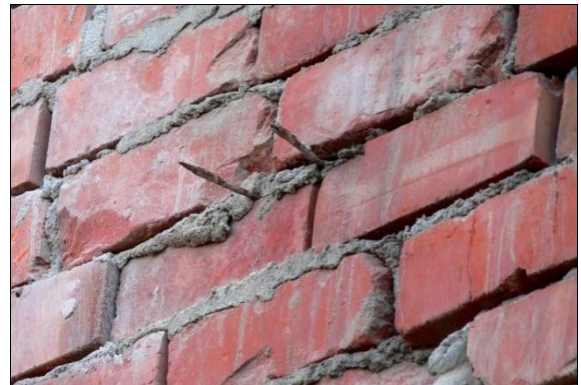
Figure 8: Deteriorated "horseshoe" shaped wire cavity tie.
