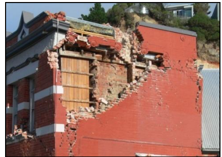
(c) Post-June 2011 – collapse of the wall
