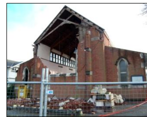
(d) Christchurch Chinese Methodist Church, overturning of the top of the whole façade
