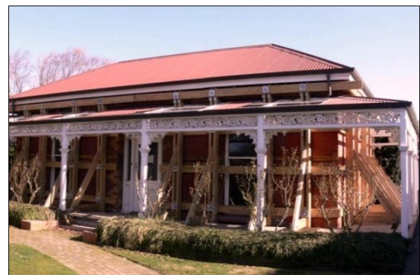
Figure 33: Extensive timber temporary shoring of a residential URM building following 4 th Sept earthquake.
