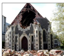
(c) Rose Historic Chapel, overturning of the top of the whole façade
