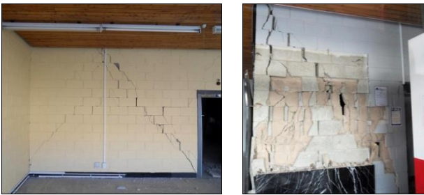
(a) Severe diagonal shear cracking of RCM shear walls (b) Close-up of diagonal shear cracking
