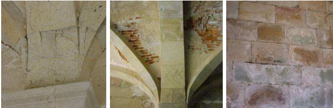
Figure 2. Examples of observed damage: (a) cracks; (b) large movements; (c) material damage and deterioration.
