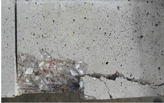
Fig.4: Spalling of SF40 after 600 \text{ }^\circ\text{C} .
