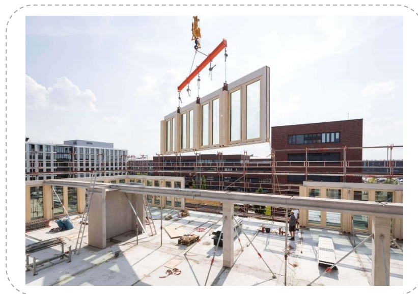
Figure 35 – How the CREE system was assembled on-site. (Sustainable building systems | timber hybrid office buildings - CREE Buildings,)
