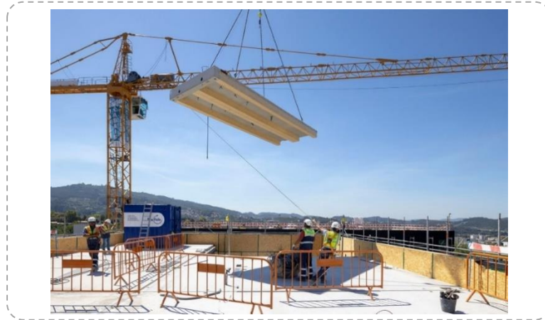
Figure 91 – Using a portable crane and a tower crane with the trained crew in the assembly process.
