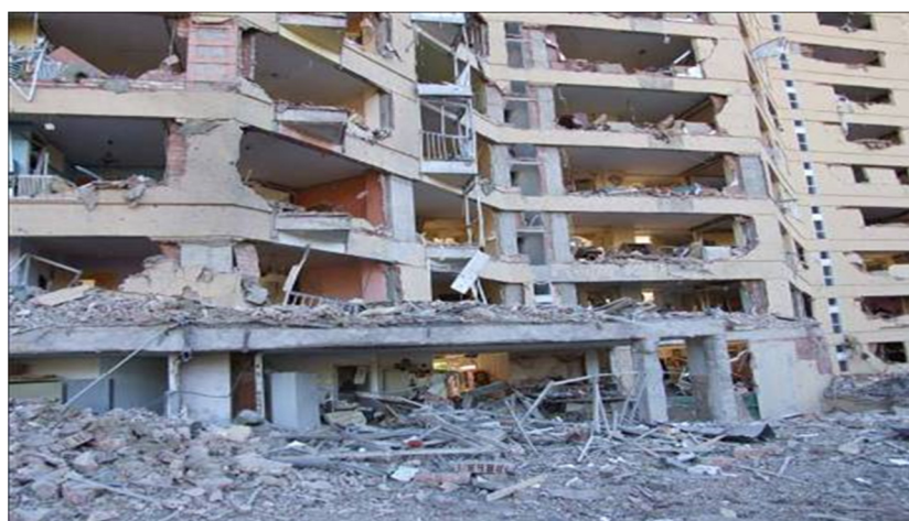
Figure 1. Structure damaged by a Vehicle-Borne Improvised Explosive Device (VBIED) explosion (Burgos, 2009).
