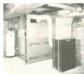
York cooler matched with gas heater.
