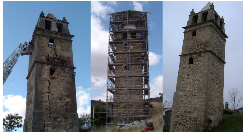
Figure 7. Overview of the Mogadouro tower before, during and after the rehabilitation works.
