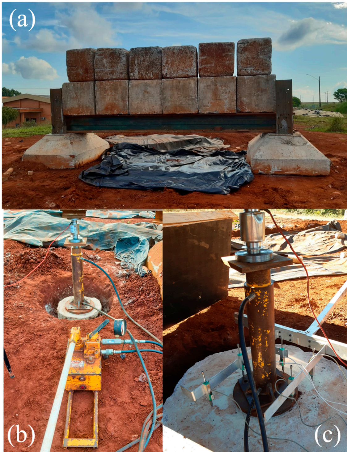
Figure 7. Load application system (a) reaction structure; (b) load application; (c) measurement of the vertical displacement.
