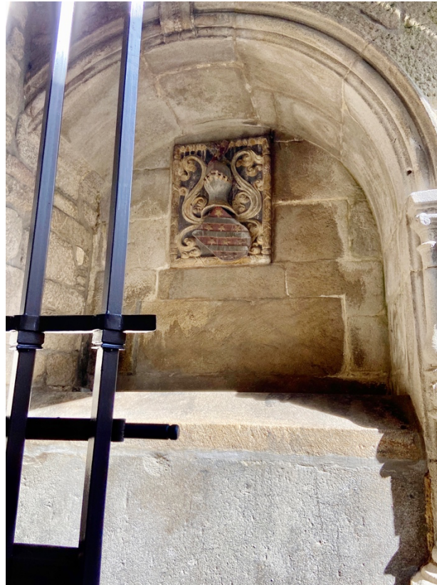
Figure 6. Chapel of Nossa Senhora das Graças , present time. Source: Photography of the author. Courtesy of Museum Treasury, Sé of Braga.
