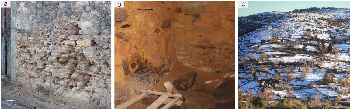
Fig. 8.1 – Examples of damage observed during the fieldwork: (a) severe salt damage on well-defined foliation schist masonry wall (livestock compartment); (b) severe salt damage on well-defined foliation schist masonry wall (wine cellar), with large amounts of disaggregated material (powdering) accumulated at the base of the wall; (c) “branda” of Aveleira (Peneda mountain range) covered with snow during the winter.
