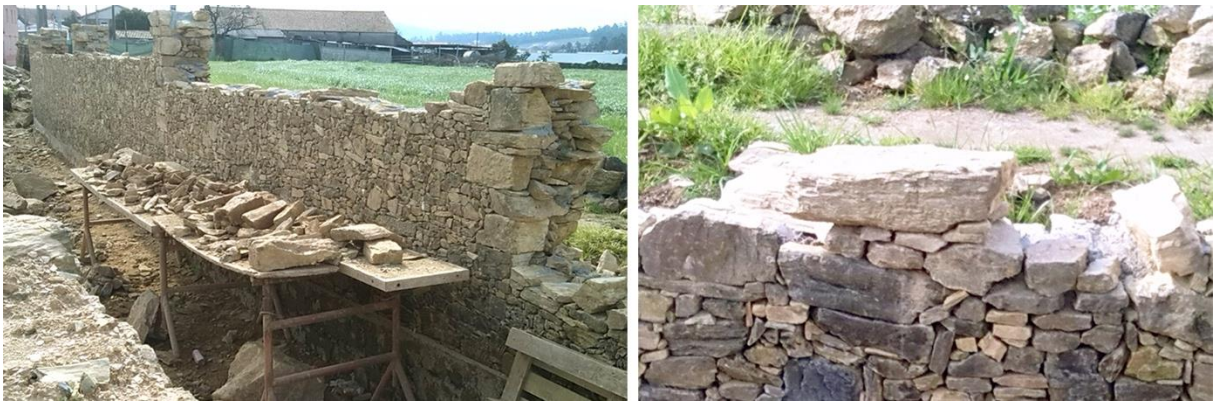
Fig. 6.4 – High farm wall under construction, with details of schist stones blocks bedded into position (S. Pedro de Rates, Póvoa de Varzim).
