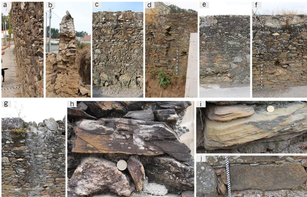
Fig. 9.10 – Examples of damage identified prior to reconstruction of the wall (see also Table 9.2).
