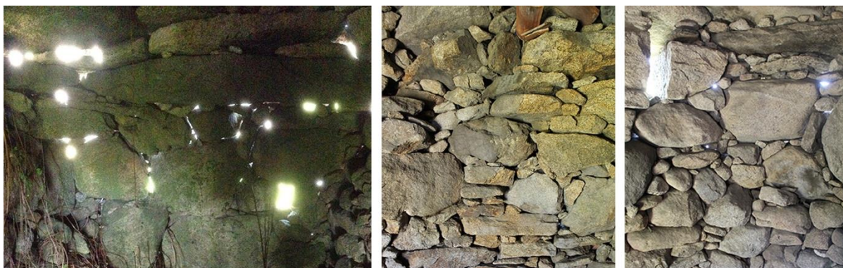
Fig. 9.34 – Examples of masonry walls' superficial textures, seen by the inside of buildings.
