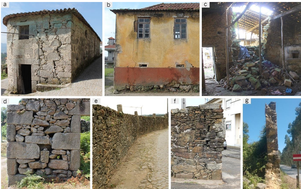
Fig. 6.13 – Some example of structural damage seen during the exploratory visits: (a) multiple cracks caused by the opening of joints (Paço Vedro de Magalhães, Ponte da Barca); (b) vertical cracks on facade with render (Laúndos, Póvoa de Varzim); (c) partial disaggregation and collapse due to push-over load caused by a roof beam (Fonte Boa, Esposende); (d) partial disaggregation of masonry superficial texture (Vale, Arcos de Valdevez); (e) high farm wall out-of-plane deformation (Barqueiros, Barcelos); (f) deformation and opening of joints crack on farm wall corner (Barqueiros, Barcelos); (g) out-of-plane deformation caused by the loss of monolithic behaviour and deformation at the base of the wall (Laúndos, Póvoa de Varzim).
