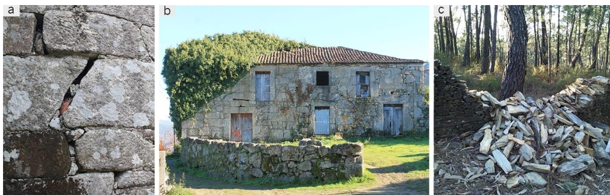
Fig. 6.14 – Examples of seen non-structural damage caused by biological colonization: (a) micro species colonization on exposed granite wall showing a large structural crack (Ermida, Ponte da Barca); (b) several smaller and a large-size specie colonizing abandoned rural house (Vila Nova de Muía, Ponte da Barca); (c) collapse on dry-stack wall caused by tree (Paradela, Barcelos).
