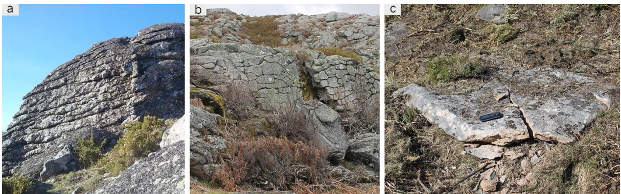
Fig. 8.3 – Examples of frost damage on granite outcrops: (a) failure along a preferred orientation; (b) fracturing of a face of granite outcrop; (c) detachment of a small platy shaped granite stone block.
