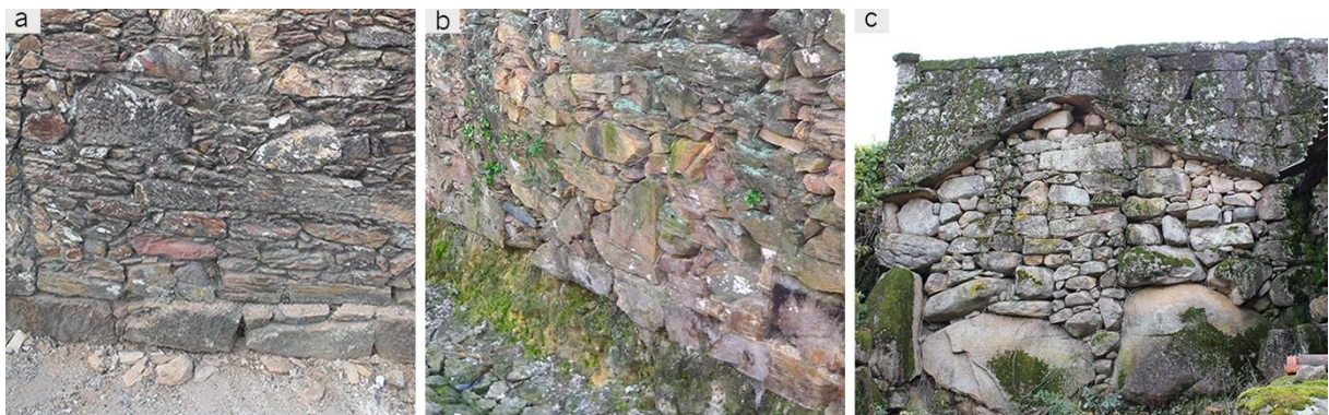
Fig. 6.6 – Examples of different types of foundations found on load-bearing walls during the exploratory visits: (a) shallow foundation, 0.05 m wider than the cross-section (Barqueiros, Barcelos); (b) direct foundation with the first row of masonry made of large stone blocks (Barqueiros, Barcelos); (c) granite massif used as foundation (Lindoso, Ponte da Barca).
