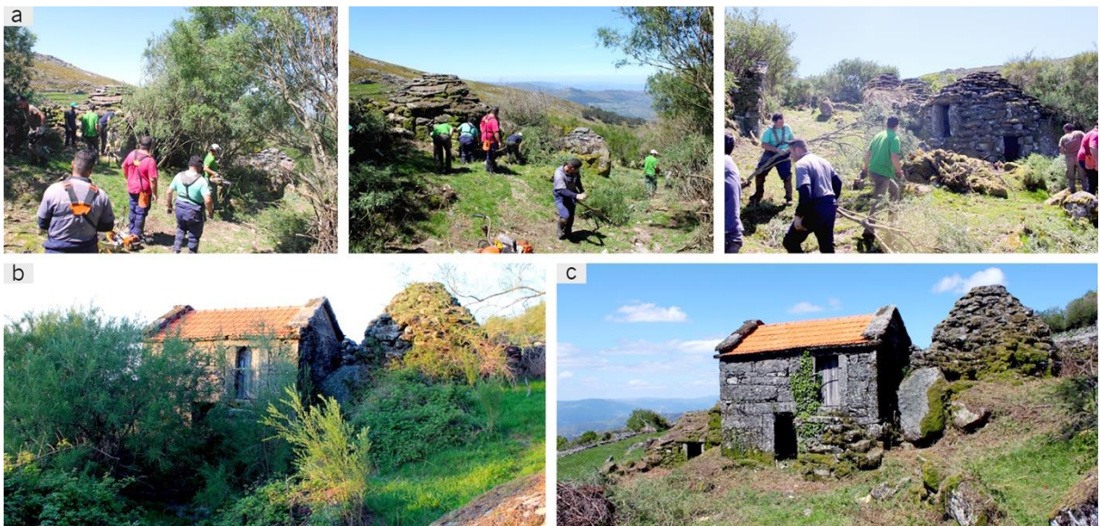
Fig. 9.23 – Images from the cleaning operation: (a) cleaning works by the Equipa de Sapadores Florestais do Gabinete Técnico Florestal do Município e da Associação Floresta Atlântica; (b) Group B before the cleaning operation; (c) Group B after the cleaning operation (photos from Fernando C. Barros).
