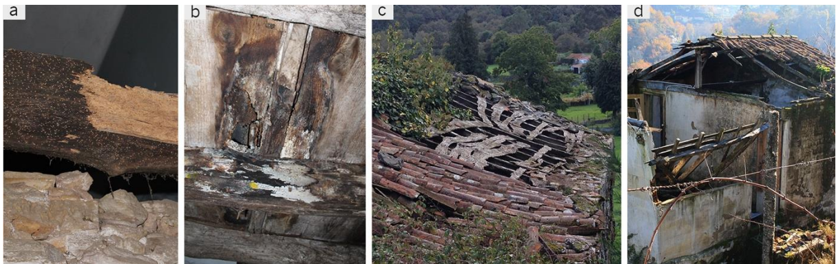
Fig. 6.15 – Examples of damage seen on timber structures: (a) insect colonization on pavement beam (Barqueiros, Barcelos); (b) rotting of timber pavement due to infiltration from the roof (Barqueiros, Barcelos); (c) decaying roof structure due to the loss of the roof tiles (Tumio, Paredes de Coura); (d) building in ruins due to collapsed roof (Vila Nova de Muía, Ponte da Barca).
