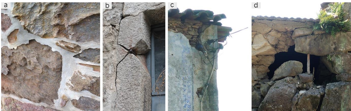
Fig. 6.17 – Some of the typical example of poor intervention on vernacular buildings found during the exploratory visits: (a) the use of incompatible materials (Barqueiros, Barcelos); (b) the insertion of metal elements on stone blocks (Ermida, Ponte da Barca); (c) new infrastructures poorly introduced (Balazar, Póvoa de Varzim); (d) unsuitable reinforcement solutions (Antas, Esposende).
