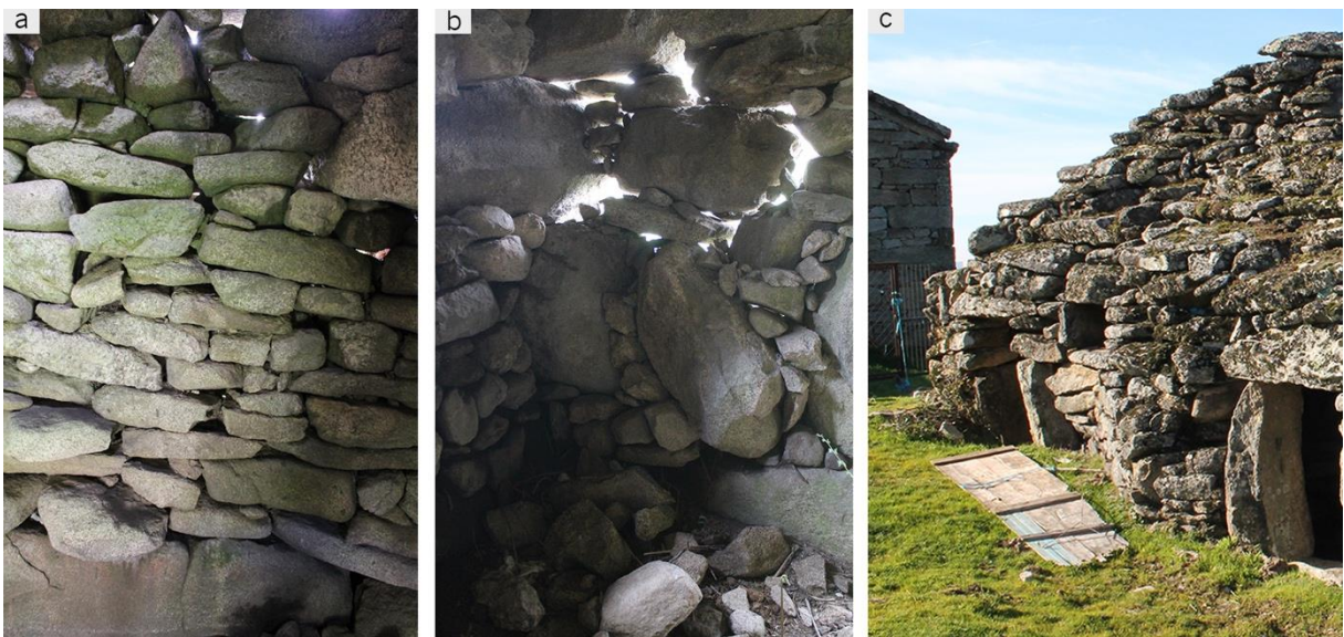
Fig. 9.38 – Masonry walls' examples of structural damage: (a) vertical cracks (opening of joints and fracture of masonry units); (b) disaggregated and partially ruptured masonry wall; (c) large masonry wall deformation.
