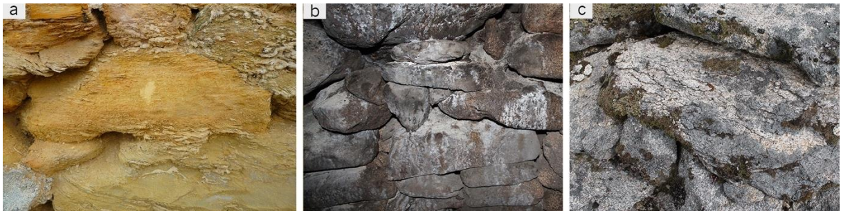
Fig. 8.2 – (a) intense powdering and lamellar disaggregation caused by salts on XL and XR schists [36]; (b) example of salt efflorescence and sanding on GE granites [36]; (c) superficial disaggregation (splintering) caused by frost damage on GE granite corbelled dome platy shape stone blocks [36].
