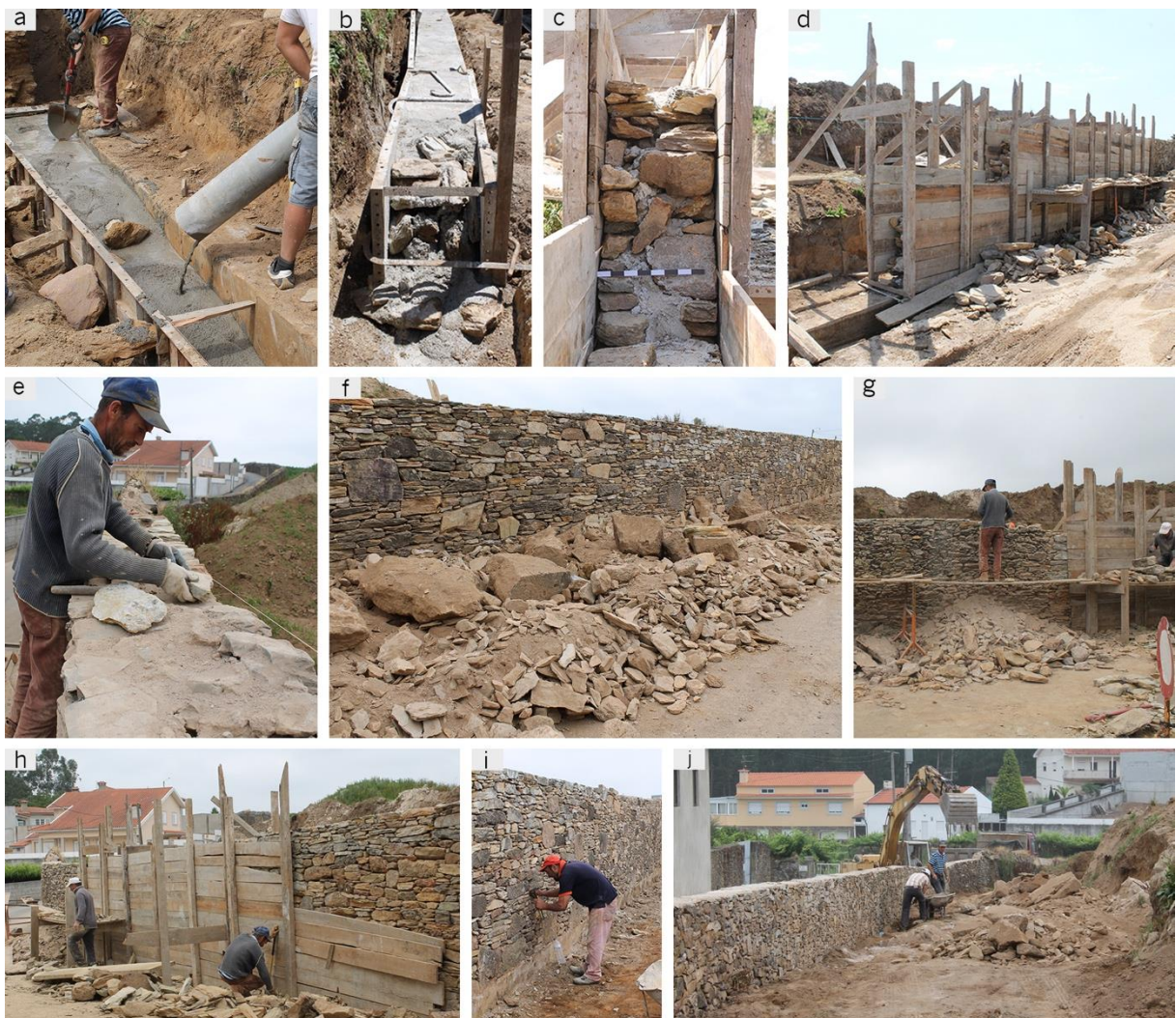
Fig. 9.12 – Different steps of the rebuilding of the farm wall: (a) and (b) shallow foundation construction; (c) cross-section of the double-leaf wall; (d) timber formwork and scaffolding; (e) bedding of a layer of stone blocks; (f) new wall and nearby materials from the demolished wall; (g) connecting of the new wall with the existent wall; (h) moving of the formwork; (i) pointing of the open joints with spalls; (j) correction of the terrain slope.
