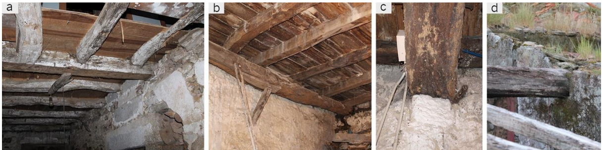
Fig. 6.9 – Examples of connections between timber beams and load-bearing walls: (a) pavement beam embedded into the wall (Barqueiros, Barcelos); (b) pavement main support beam embedded into the wall, and supporting secondary beams (Santa Maria of Bouro, Terras de Bouro); (c) pavement support beam supported over a "cachorro" (Santa Maria of Bouro, Terras de Bouro); (d) roof beam embedded into the wall (Barqueiros, Barcelos).
