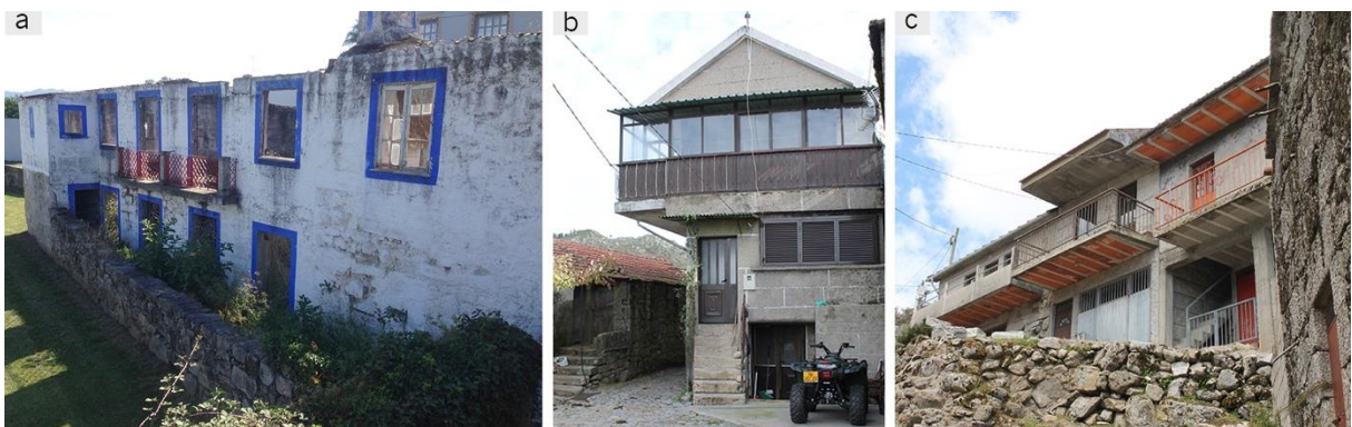
Fig. 6.16 – Examples of human caused damage over vernacular heritage: (a) state of ruin caused by abandonment (Arcozelo, Ponte de Lima); (b) loss of authenticity and identity of vernacular building due to poorly planned changes (Padrão, Arcos de Valdevez); (c) “branda” loss of identity due to the introduction of foreign models and building materials (“branda” of Gorbelas, Arcos de Valdevez).
