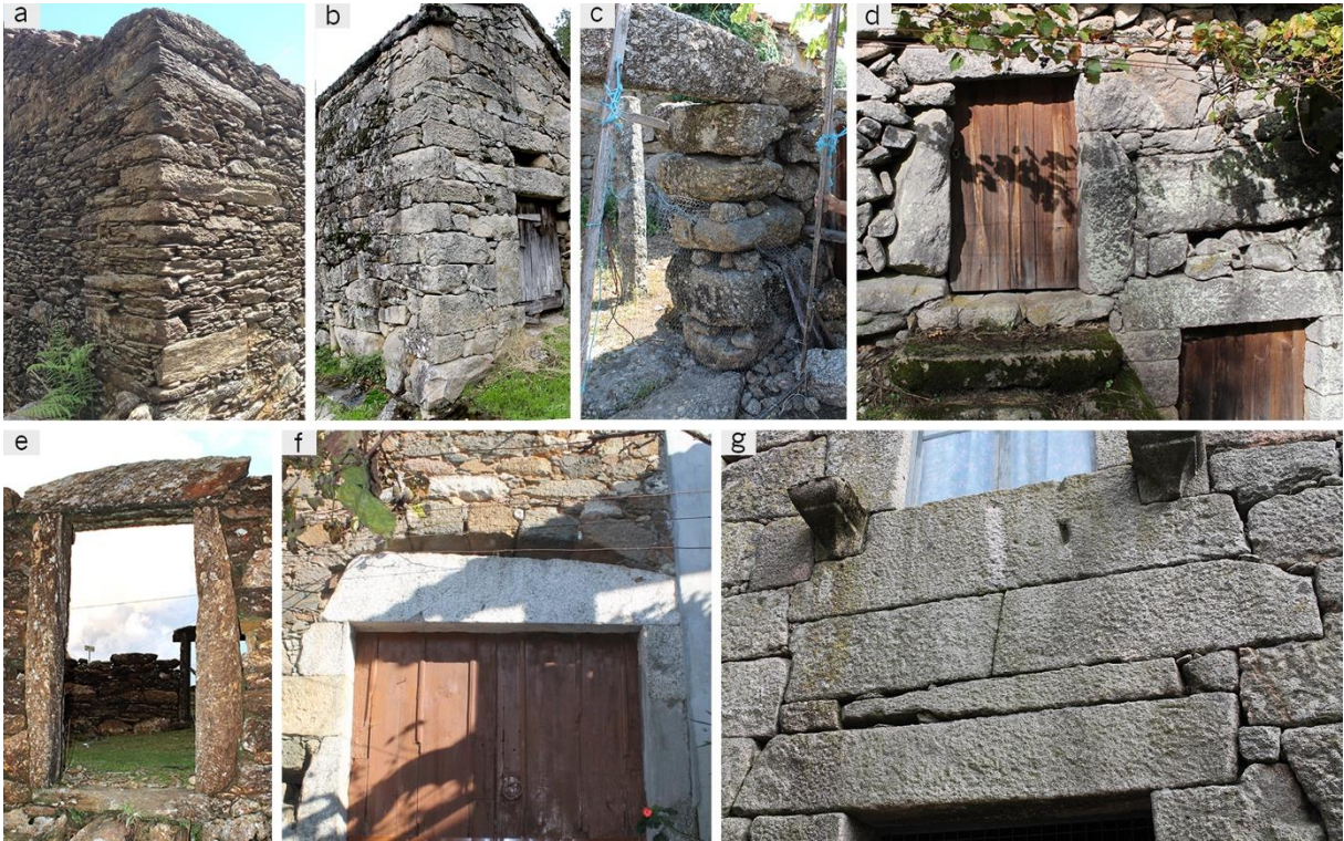
Fig. 6.8 – Examples of load bearing walls' fragile points improvements: a and (b) improvement of schist and granite different load-bearing walls on corners (Agra mountain range, Viana do Castelo; and Padrão, Arcos de Valdevez); (c) improvement of vertical edges with bondstones (Vale, Arcos de Valdevez); (d) improvement of vertical edges with large-size and irregular stone blocks and jamb stones (Lindoso, Ponte da Barca); (e) improvement of vertical edges with large-size schist stone blocks (Agra de Cima, Caminha); (f) lintel protected by an arch (Paradela, Barcelos); (g) lintel protected by a flat arch (Ermida, Ponte da Barca).
