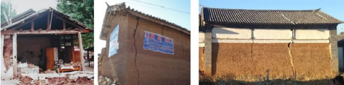
Figure 13 - Mostly observed damages in rammed earth building subjected to earthquake (Wang et al. , 2016)
