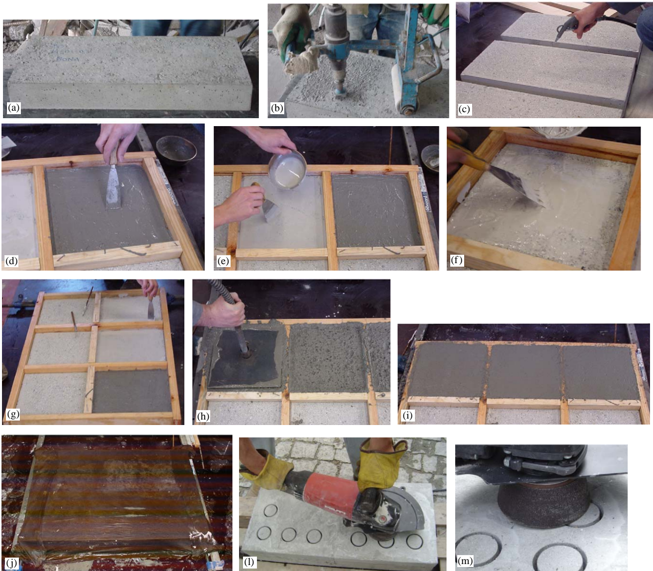
Fig. 1. Main steps of the bond process of the SFRC overlay: (a) the specimen surface before roughing, (b) the rough machine used, (c) cleaning the top surface with compressed air jet, (d) placing the bond product P3, (e) placing the bond product P2, (f) placing the bond product P1, (g) overview of the bond coats before casting the fresh SFRC overlay, (h) consolidating of the SFRC, (i) final aspect of the finished surface, (j) curing with wet burlap, (l) overview of the machine for removal of a very thin layer from the concrete surface, and (m) detail of the stone wear device.
