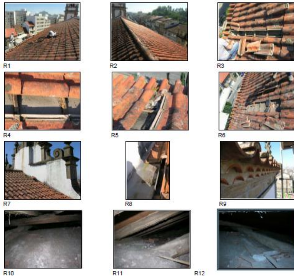
Figure 47 - Photographic survey on the roof by architect Francisco Perry Azeredo (Betzer et al., 2014).
