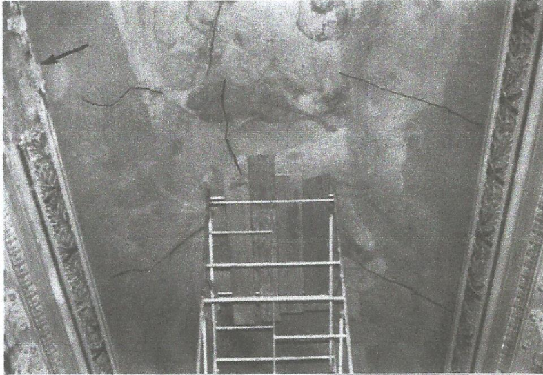
Figure 50 – Cracks in the vault over the foyer (Schiros, 1975)
