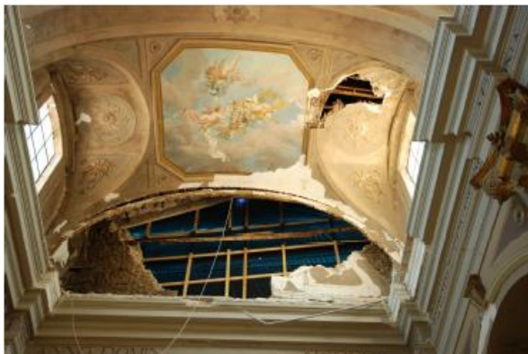
Figure 18 – Partial collapse of the barrel vault in Saint Biaggio Church from L'Aquila earthquake (Binda et al., 2010)
