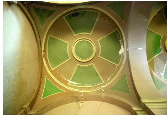
Figure 19 – Circular cracks in spherical vaults of lateral naves in Saint Biaggio Church from L'Aquila earthquake (Binda et al., 2010)
