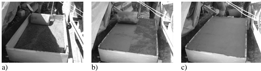
Figure 4.21. Execution of sand cement layer: a) first stage compaction; b) final compaction; c) layer after final compaction
