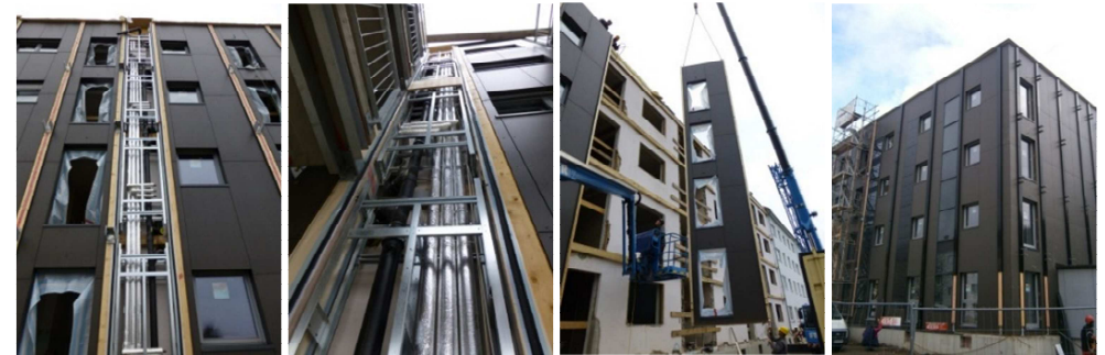
Different steps of the building renovation process: installation of the building services, assembling of the prefabricated façade modules, almost finished building envelope (f.l.t.r.)
