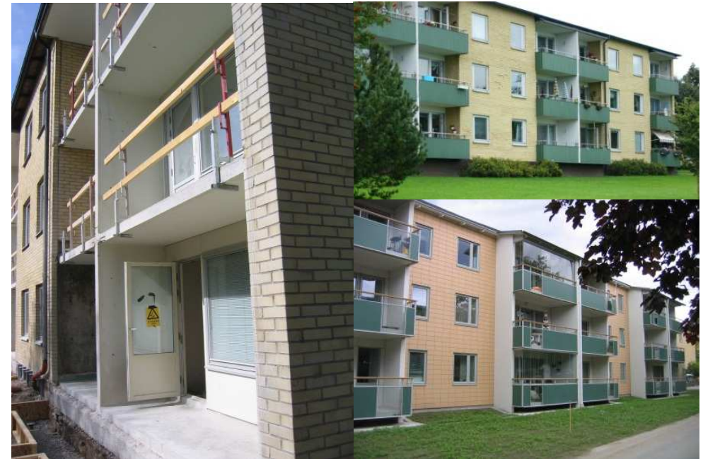
Long side façade with balconies before (left and above) and after (below) renovation.
