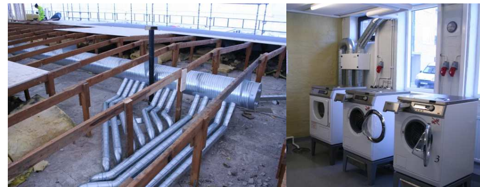
Installation of ventilation ducts in the new attic and new washing machines in the common laundry room.
