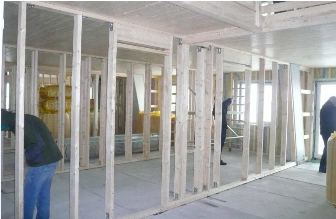
New internal walls and inserted deck at the first floor of block B.
