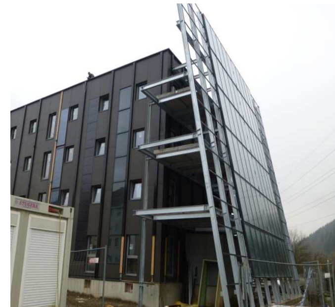
Solar thermal and PV panels on the south facade
