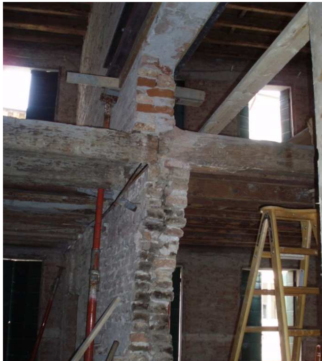
Crooked walls, before renovation
