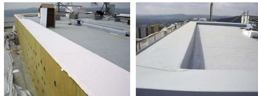
The attic during the renovation - installation of additional thermal insulation over the attic to reduce the thermal bridge (left) and a view of the new waterproofing/covering layer made of mPVC sheets (right). Precise design and construction of structural details are crucial for proper function of any energy efficient building. [1]
