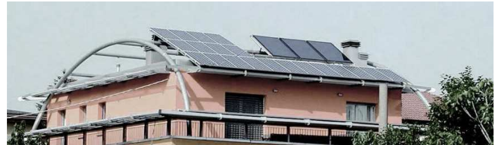
Solar and photovoltaic panels.
