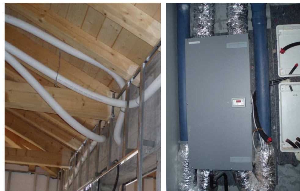
Mechanical ventilation system
