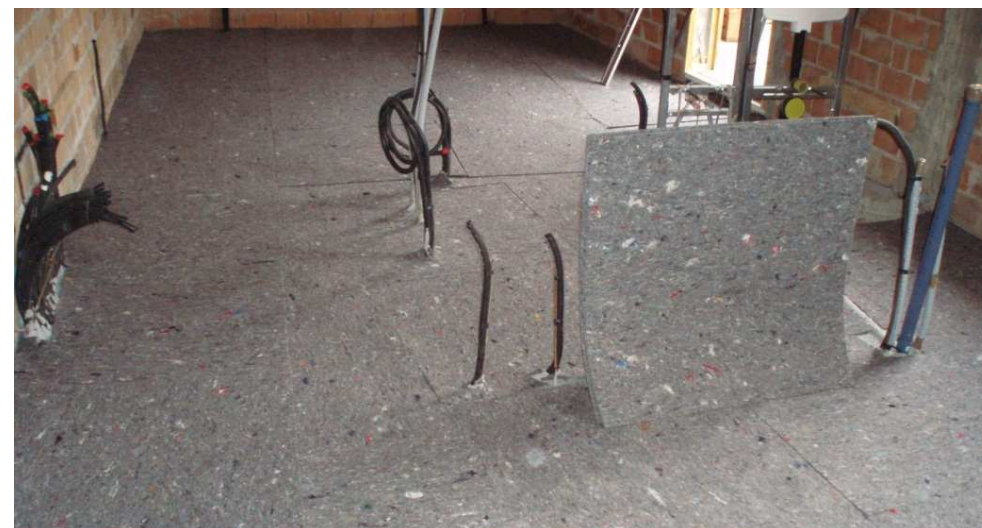
Photovoltaic system - TNT under flooring above systems
