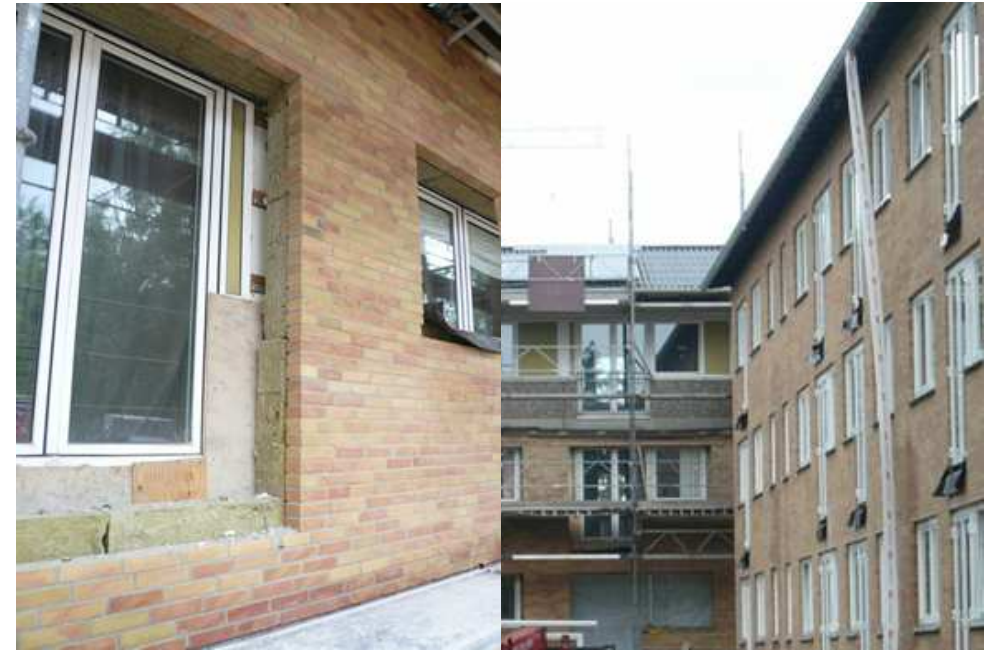
190 mm insulation plus exterior solid standard bricks. Energy windows – aluminium – wood, 3-layer energy glass. In the panel walls: 285 mm insulation plus exterior solid standard bricks.
