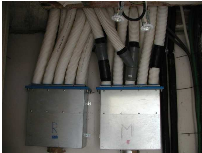
Distribution section of mechanical ventilation system.
