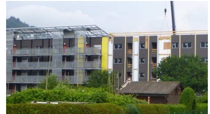
Left building part already renovated – right building part in the middle of the renovation
