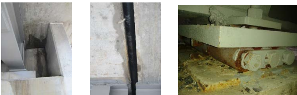
Fig. 3. Water leakage – cause to corrosion consequence
