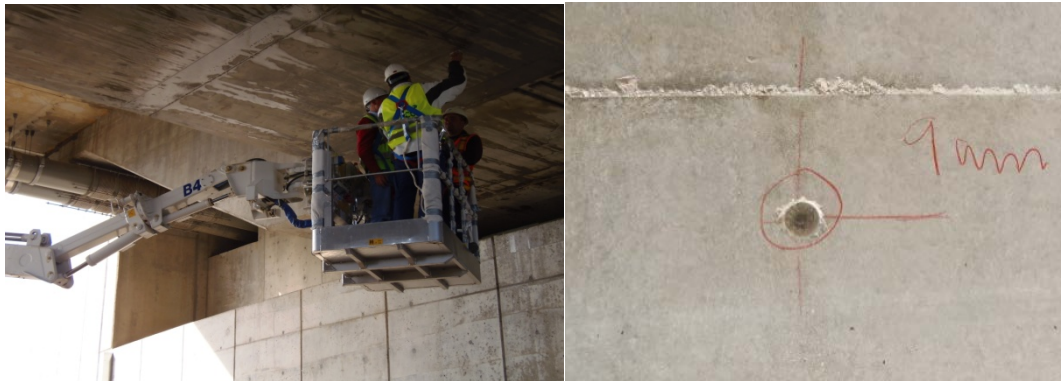
Fig. 2. Left: On-site measurement of resistivity in the segments after watering. Right: Checking the concrete cover.
