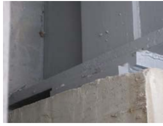
Fig. 4. Direct contact between the steel girder and back abutment wall
