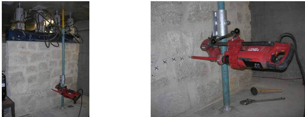
Figure 5-48 Core drill setup for the single tube-jack test in the irregular wall
