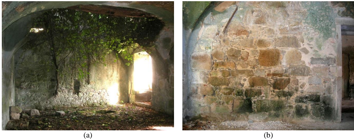
Figure 7-3 “The fig tree room”: (a) branches from the fig tree coming through the collapsed ceiling on the north side of the room; and (b) the south wall of the room where the tests were performed
