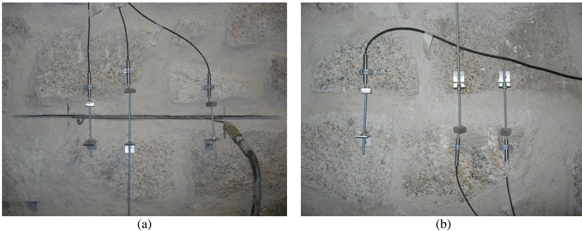
Figure 5-53 Complete test setup for the single flat-jack test in the irregular wall with the flat-jack inserted in the slot and LVDTs attached: (a) front of the wall; and (b) back of the wall
