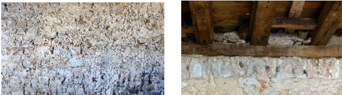
Figure 36: Current state of Central Building. (Left) Morphology of stone masonry wall; (right) timber floor beams on transversal timber plate (credits: J. Ortega).
