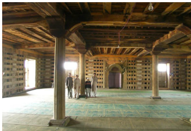
Figure 23: Cribbage construction system. The interior is clad with plywood in this photo (credits: R. Langenbach).
