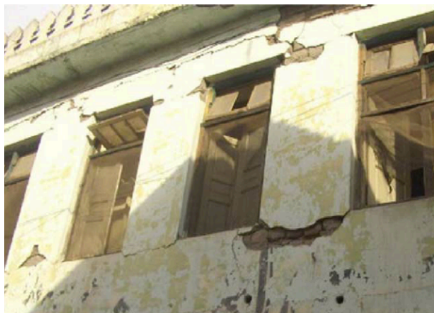
Figure 3: Rocking failure of masonry pier in 2005 Kashmir earthquake (credits: Javed, 2008).
