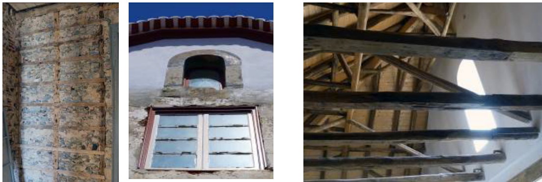
Figure 35: Current Condition. (From left to right) timber partition wall; new gable at the back of Central Building; and reconstruction of mansard roof (credits: J. Ortega).
