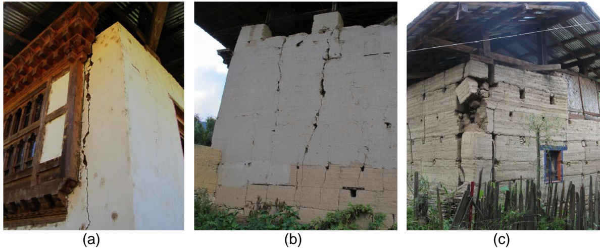
Figure 10: Typical damages of RE constructions (a) Separation of corner walls; (b) vertical wall cracks and (c) corner failure
