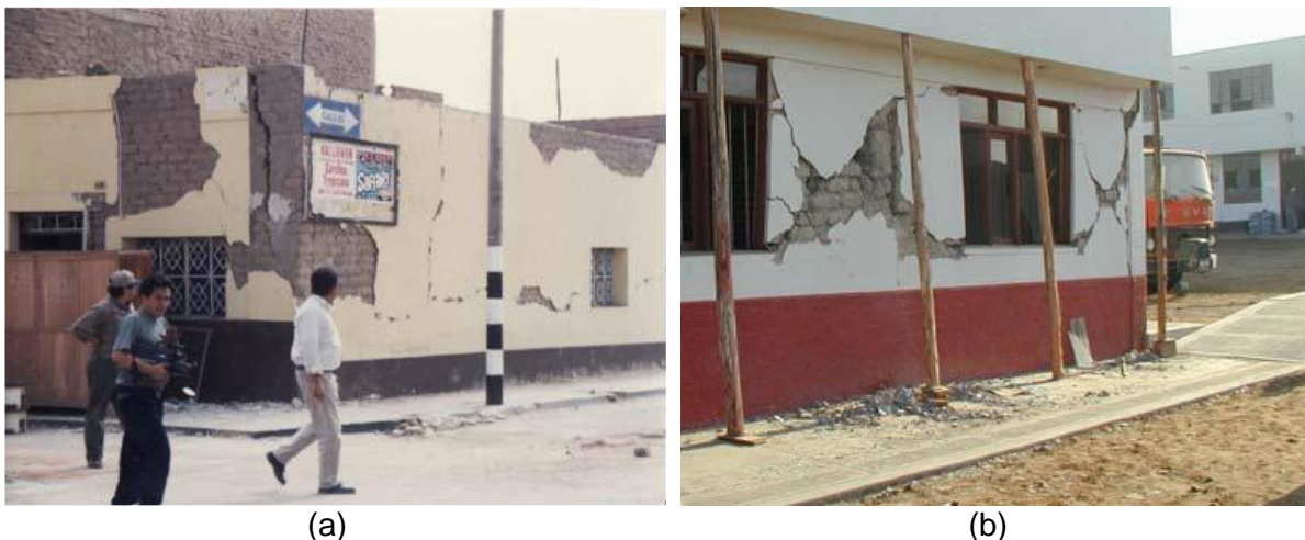
Figure 6: Adobe houses with seismic damage (a) Vertical cracks at corner of front wall and (b) Diagonal shear cracks (Blondet & Aguilar, 2007)
