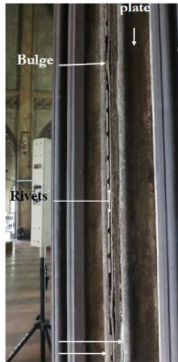
Figure 34 – Bulging at the column.
