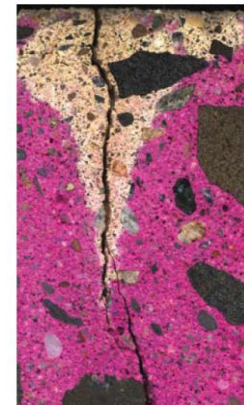
Fig. 4: Lapped cross section of concrete showing carbonation flanking a 2.5 in. (65 mm) deep vertical crack. The V-shaped carbonation zone does not extend to the end of the crack
