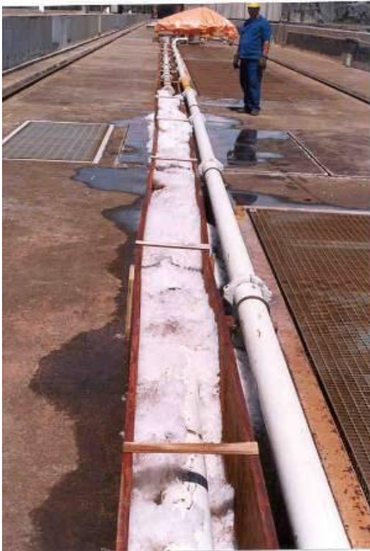
Steel tubes covered with ice at the 2 nd stage Itaipu HPP (2003)
