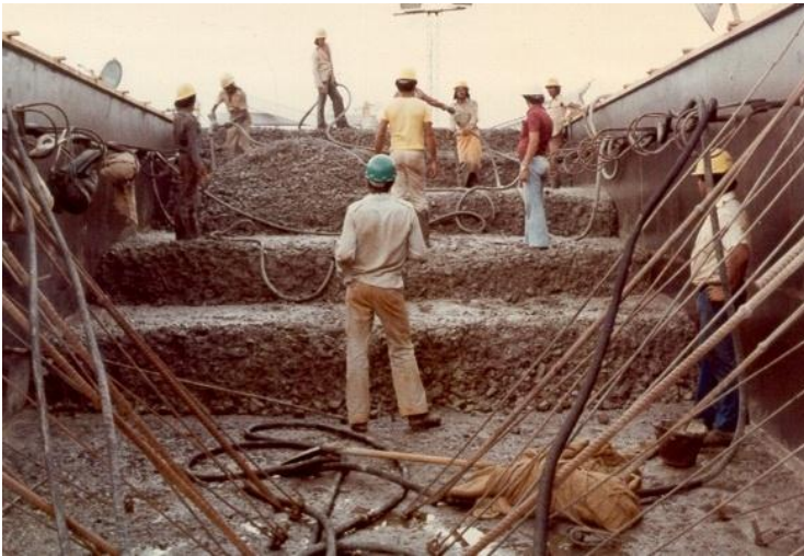
Conventional concrete (CVC) block construction with 2m lift height and 0,5m high sub lifts (HPP in Brazil).
