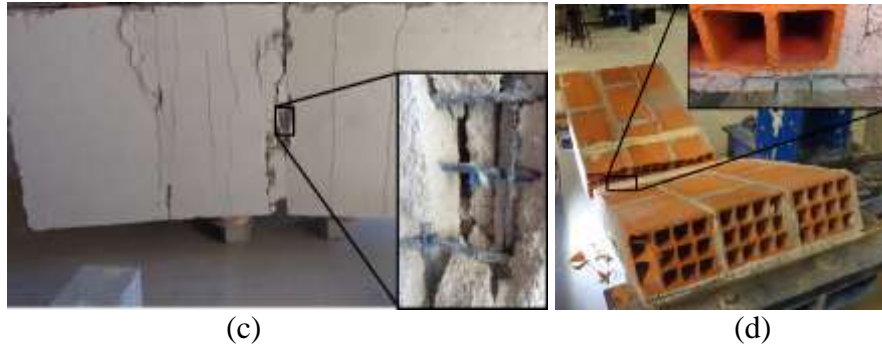
Fig. 24 - Typical failure observed in brick masonry specimens strengthened with: (a) commercial carb mesh; (b) manufactured carbon mesh; (c) manufactured glass mesh; (d) commercial glass mesh
