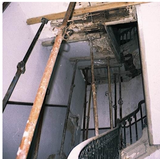
Figure 2 - Need for propping
