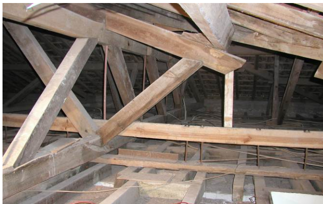
Figure 7 - Missing part of the structure due to previous interventions
