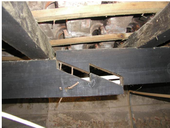
Figure 12 - Lack of contact and failure of the joint
