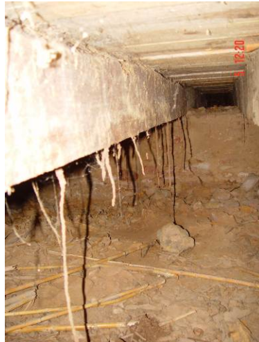
Figure 9 - Subterranean termites attack
