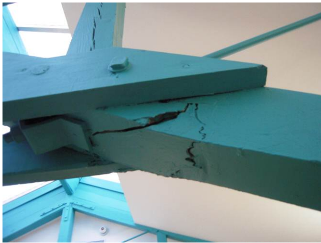
Figure 6 - Timber failure in the vicinity of the joint
