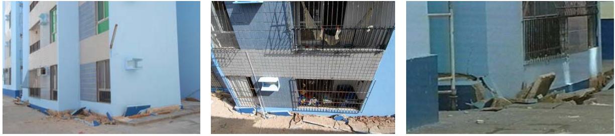
FIGURE 1 Views of the building after the collapse.
