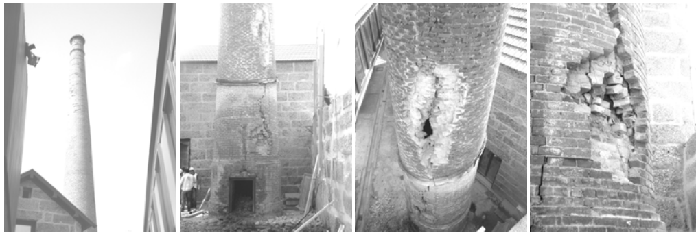
Figure 1. The Chimney and the severe openings caused by the lightning.
