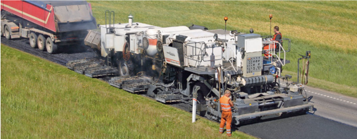
Figure 5 – Example of a hot in-situ recycling operation (adapted from adapted from Wirtgen (2013))
