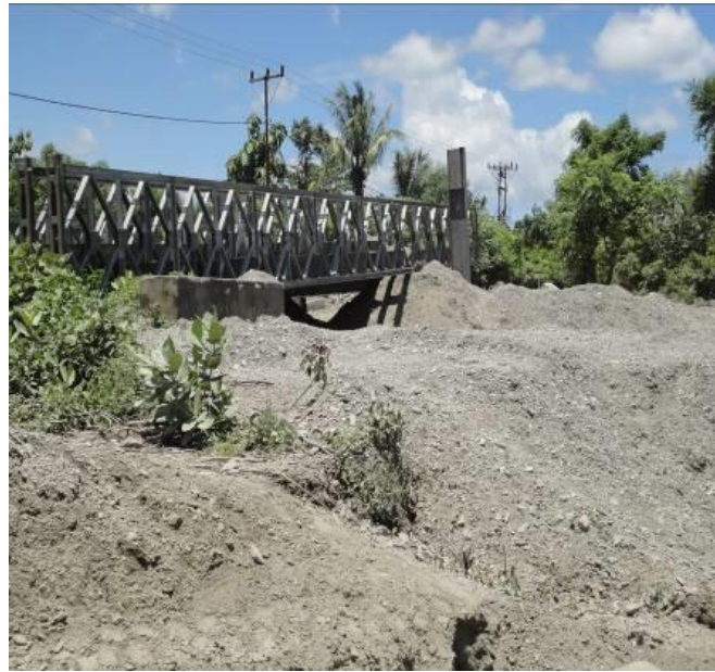
Picture 2 – A broken bridge in Liquiçá
