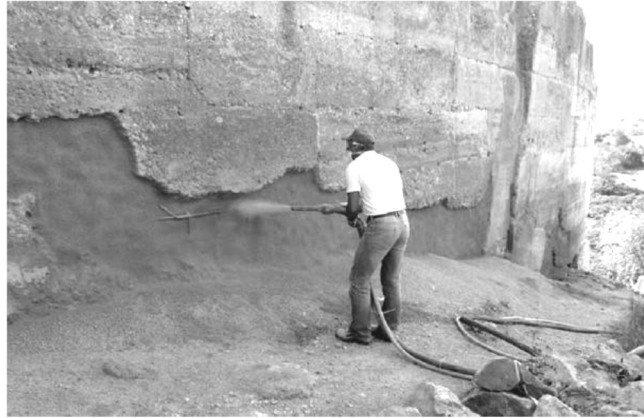
Figure 2.15 – Repair of the basal erosion of Paderne’s Castle by projecting earth at high speed (Costa et al. 2008).
