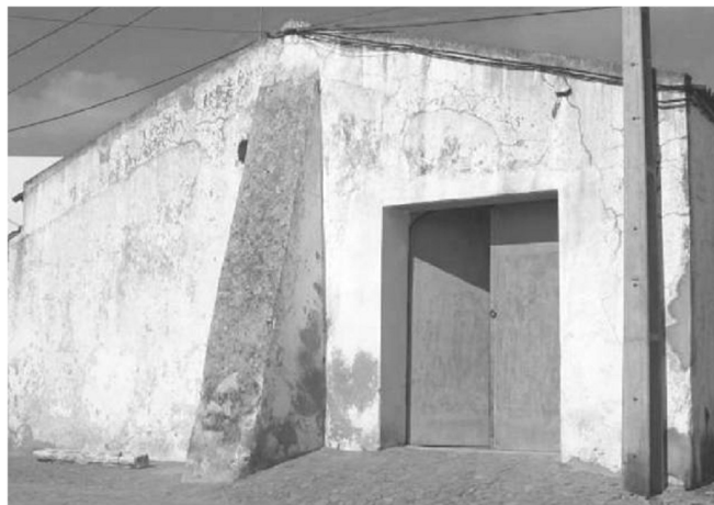
Figure 2.17 – Strengthening of a rammed earth construction by introduction of buttress in Vila Alva, Alentejo (Parreira 2007).
