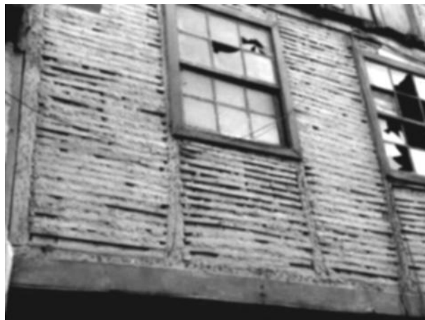
Figure 2.8 – Wattle-and-daub (“ tabique ”) exterior wall of a house in Douro North Valley Region, Portugal (Pinto et al. 2010).
