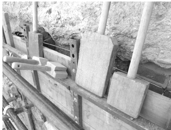
Figure 2.14 – Repair of the basal erosion of Paderne’s Castle by compacting new rammed earth material in place (Costa et al. 2008).
